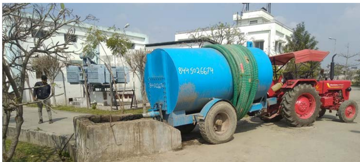
Figure 4: Private vacuum tanker discharging FSS into a chamber connected to MPS in Kargi STP
